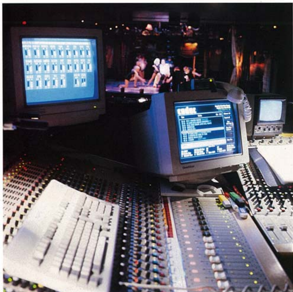
The 59-channel Cadac J-type installed for Moby Dick at the Piccadilly Theatre, London. photos: Carlos Olms
