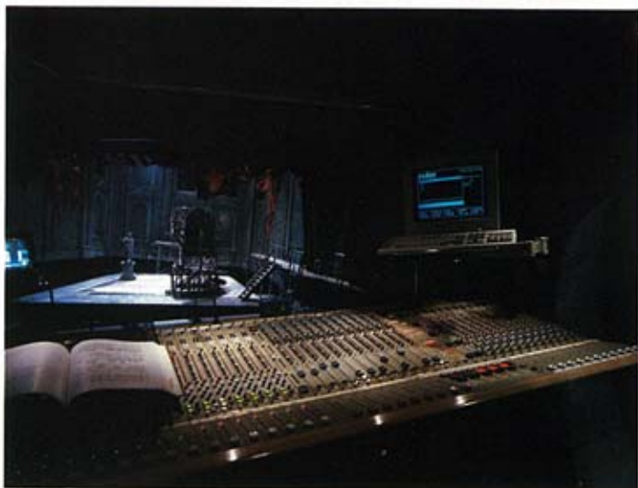
The English National Opera has recently installed a Cadac sound desk in its control position, seen here at the rear of the auditorium.
